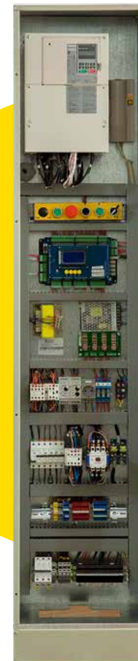
ARM Control Cabinet
